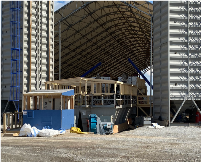
Photo 28: Paste Backfill Batch Plant and Mixing
