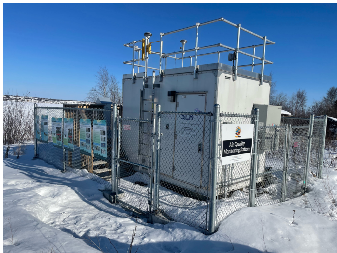
Photo 8: Air Monitor Filter and Station
