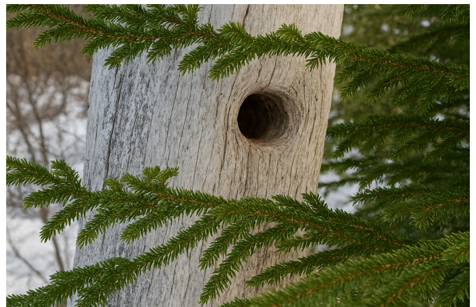
Photo 40: Woodpecker Nesting Cavity on Power Pole 2023
