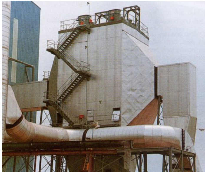
Fig 8 An example of a large electrostatic precipitator in use at a power station (cleaning a large volume gas flow)
